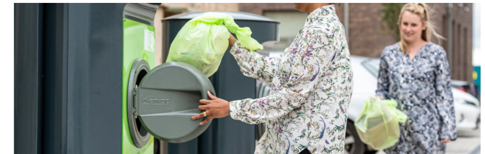
Envac System in Barking Riverside
